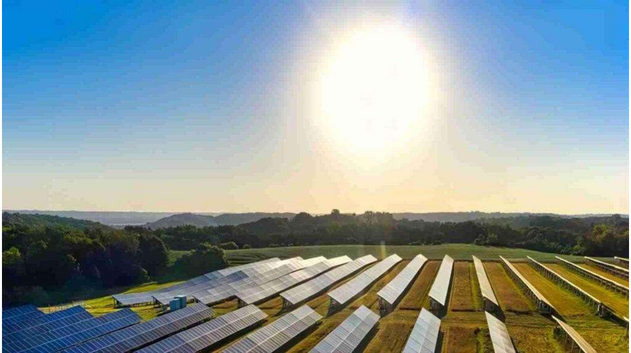
Figure 11: Typical Arrays oriented True North, with low angle setting sun in the west
